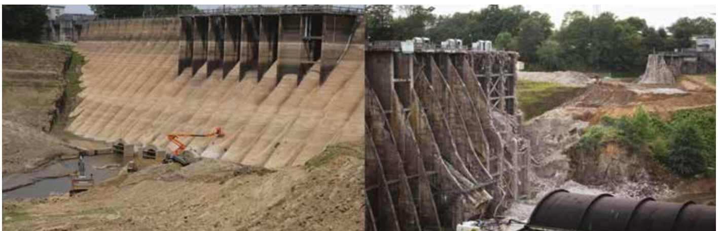
Removal of the Vezin dam in France (Selune River). The dam was 35 meters high and 200 meters wide. The removal was completed in November 2020. Pictures from European Rivers Network, one of the Dam Removal Europe partners.
